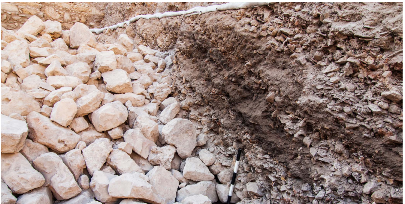
A section of the Giva'ti Parking Lot glacis, wherein the layers of the glacis' formation are clearly represented (Courtesy of Ayala Zilberstein)
